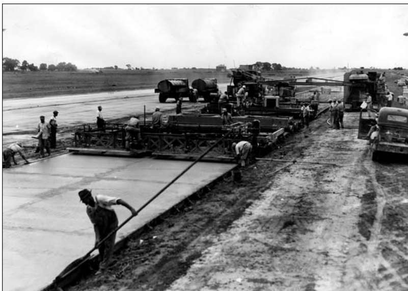
The three pictures above are of the Decatur Airport project. Summer of 1945
