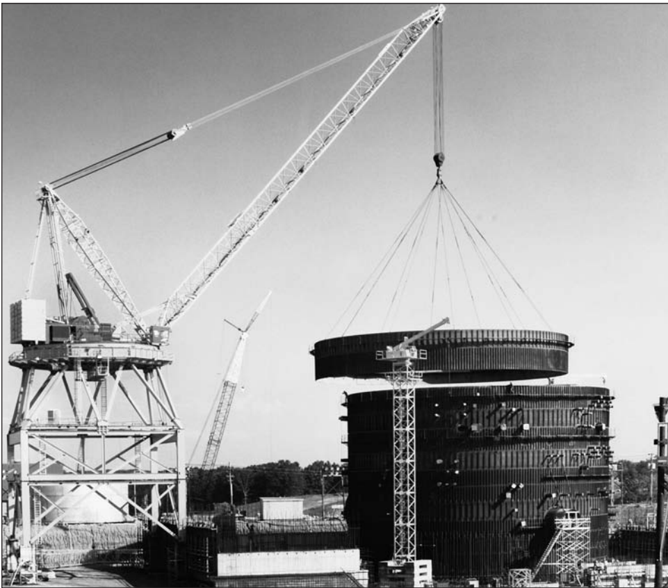
Clinton Nuclear Power Station — 1978 Brother Don Ator setting the containment walls with a Manitowoc 4600 Series B&C
