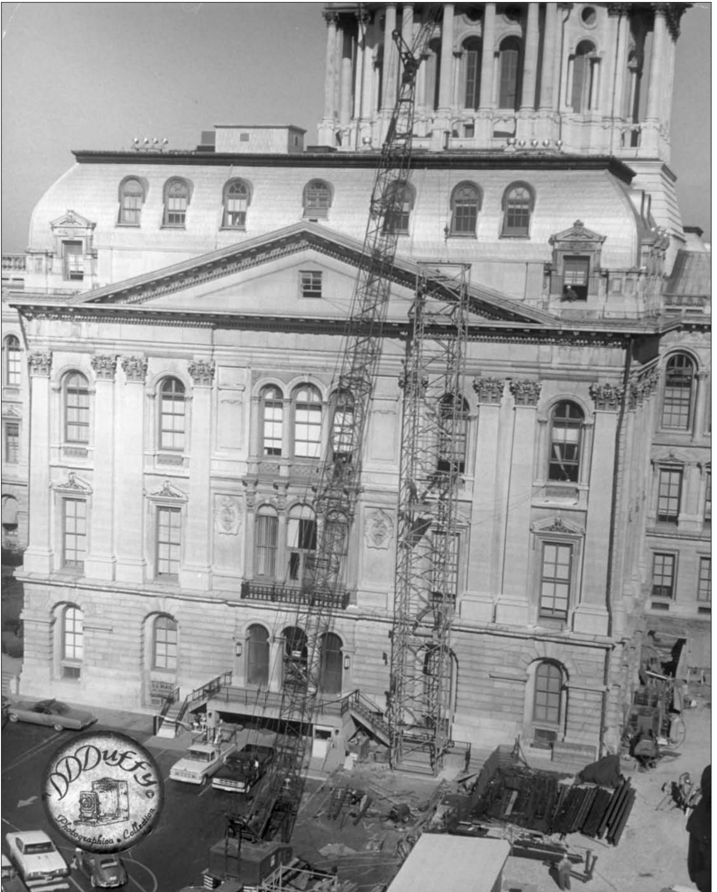
Illinois State Capitol Building Remodel — circa 1970-71 R.D. Lawrence Construction Company — Robert Lee, operator and John Bartelow, oiler
